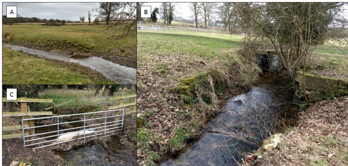
Caption 3.4 Photos of additional morphological pressures on the surveyed reach of Cantley Stream. (A) Bank erosion due to poaching by sheep on the right bank; (B) Collapsing brick wall bank protection downstream of the Cantley Stream Pond; (C) Partial blockage of the channel due to debris build up behind a gate crossing the channel.
